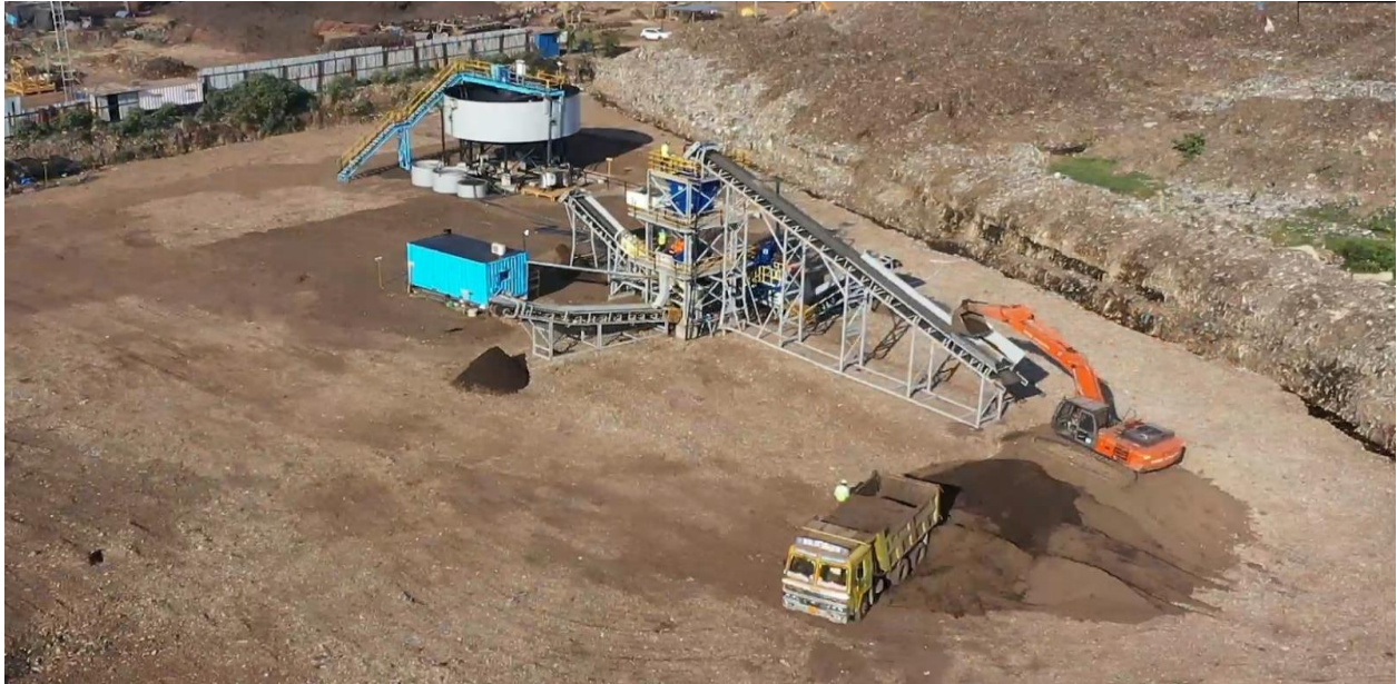
Photograph of Zigma's Sand washing unit at one of the Biomining Facilities
